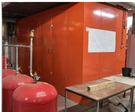
Figure 11-6. Combined Heat and Power system enclosed in sound absorbing cabinet
