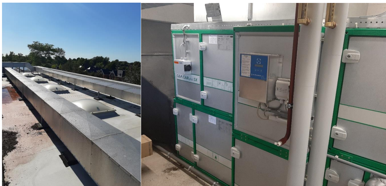
Figure A-2-1. Ducts on the roof; view of air handling unit in technical room.
