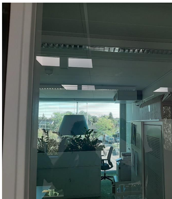
Figure A-2-4. Wall fan coil unit in south facing office
