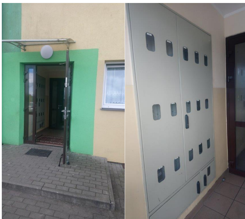
Figure 8-5. Main switchgear at the building entrance
