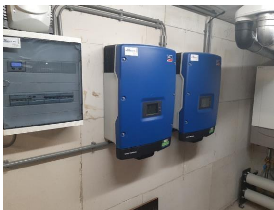
Figure A-2-6. Inverters in technical room
