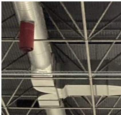
Figure 11-7. Air distribution in Expo1, in red the air supply of Expo 1 can be seen
