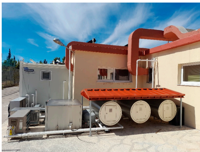
Figure 4. Outdoor horizontal water tanks under the shade. From left to right: virtual BTES, solar buffer, and space buffer tank.
