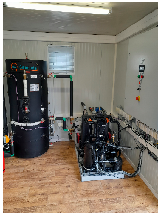
Figure 3. Heat pump and its electric/control panel in the control room next to the DHW tank.
