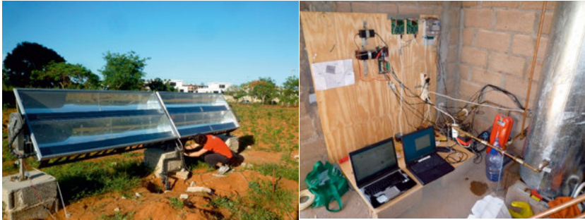
Figure 69. The C-T and C-PVT solar collectors installed in the solar tracker (left) and the installation equipment inside the laboratory housing.
