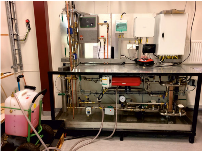
Figure 140. Hydraulic rig apparatus station with a pumping station for adjusting the temperature of the heat transfer fluid and fixing the flow rate equipped with several pneumatic valves and mixing circuits.
