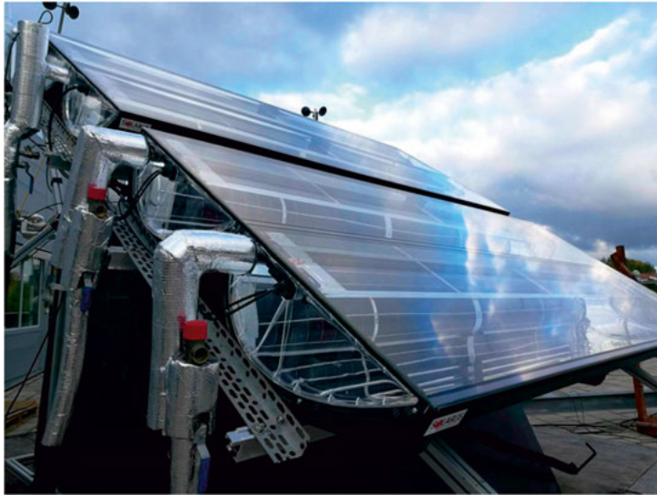
Figure 118. The Solarus Power Collector installed at Dalarna University
