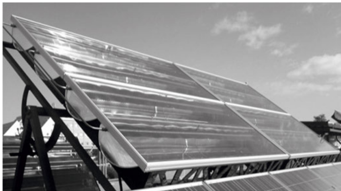
Figure 58. Four Solarus stationary concentrating thermal collectors installed at Lund University.
