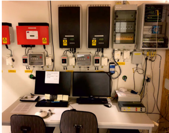
Figure 142. Solar laboratory analysis station.
