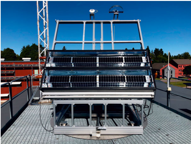
Figure 143. The DM C-PVT collector installed at the HiG solar laboratory. (V11)
