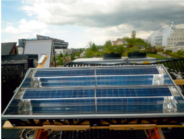
Figure 57. The first Solarus C-PVT Prototype (V0) installed at Lund University.
